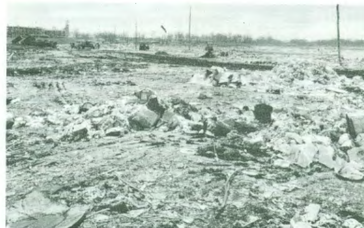
Garbage on which Pelham Bay Park's engineering marvel, Orchard Beach, was built awaits burial during construction in mid-1930s. The shell of the beach's pavilion is visible in upper left corner.
